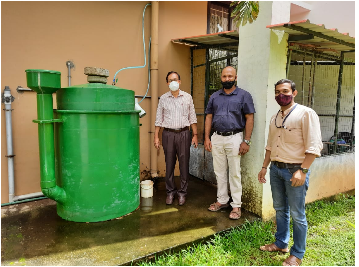
Biogas plant installed at CoF Vellanikkara, under NAHEP CAAST Project
